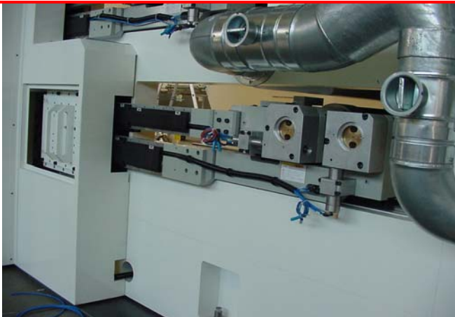
Doors And Guards Not Installed
